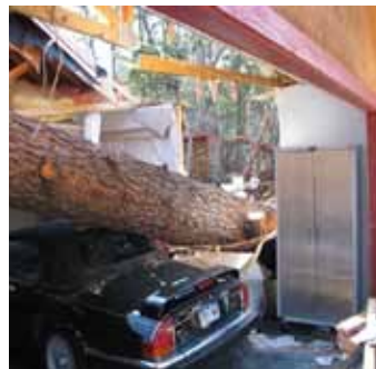
A Downed tree impacts both garage and vehicle.
